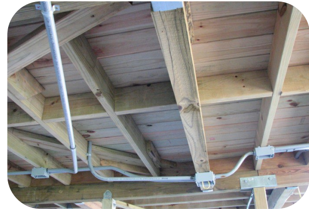
Wire, Conduit, and Bollards
