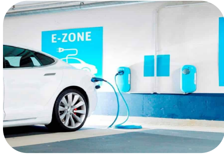
Electric vehicle supply equipment (EVSE)
